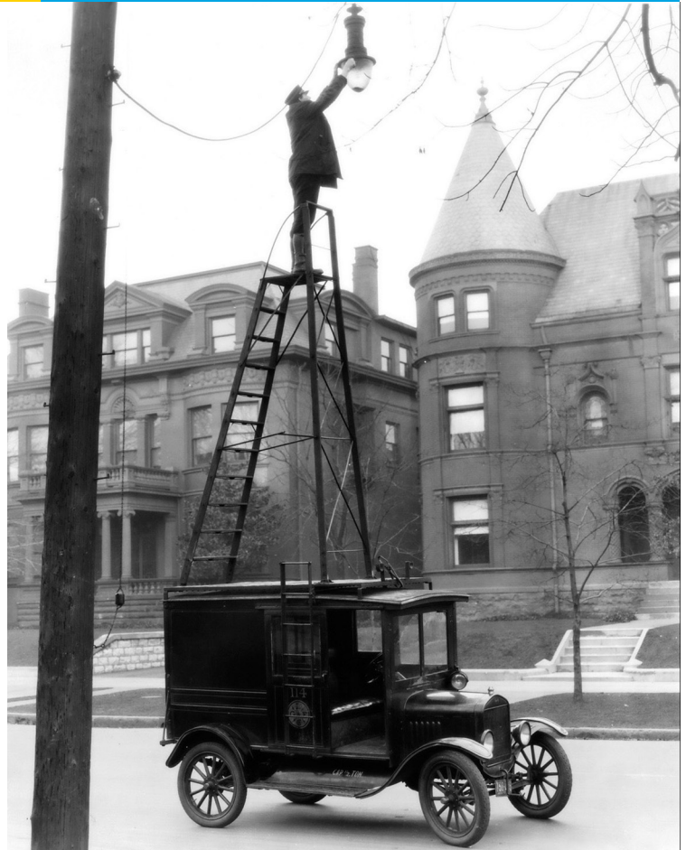
Concerns about lifetime and maintenance have been around for a long time. Credit: Ford Motor Company
